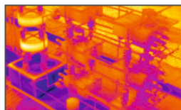
Electric Equipment Inspection
